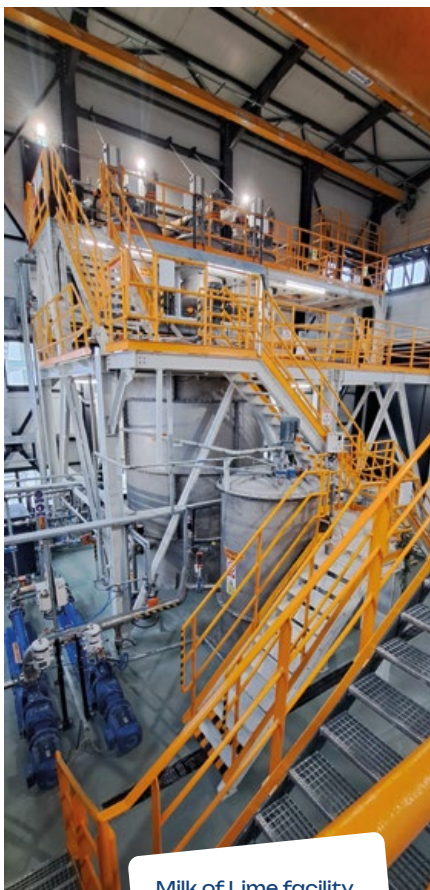
Milk of Lime facility
