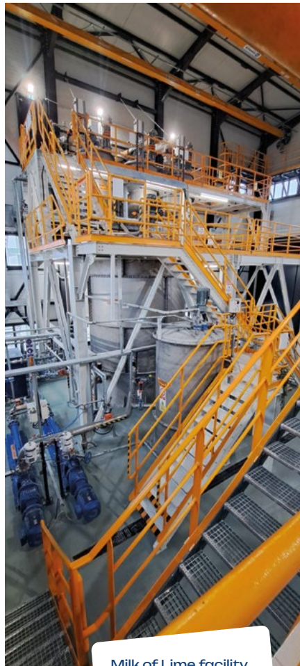
Milk of Lime facility
